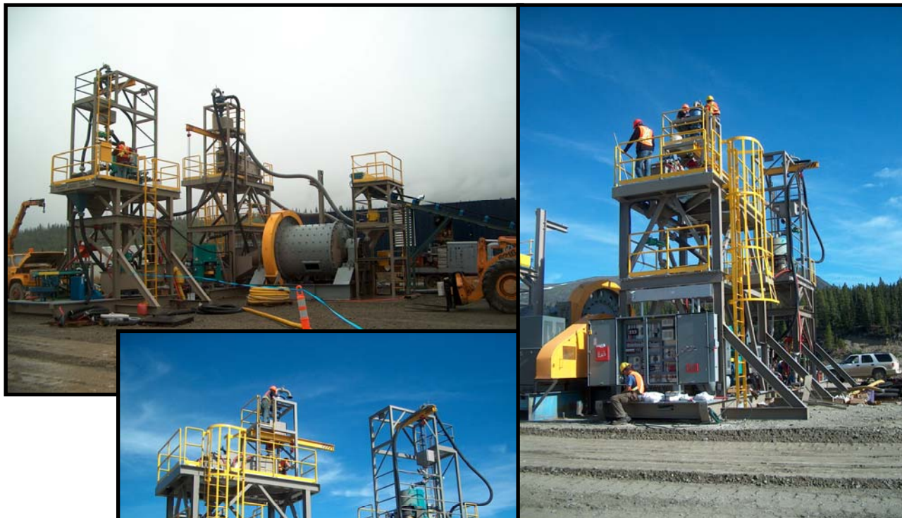
FIGUER 6-4: Photos of Grinding Mills and Gravity Concentrating Processing Plant
